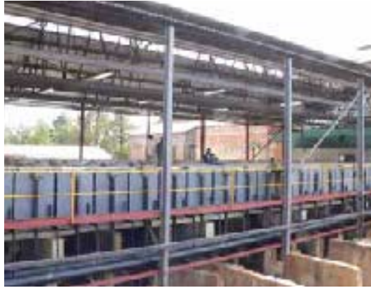
Sable copper electrowinning tankhouse
