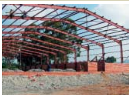
Construction of Cricket Arena on Fields College premises in Rustenburg, funded by Sun City.
