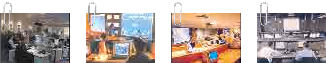
Dimension Data’s Network Operations Centres in the UK, South Africa, Singapore and the US
