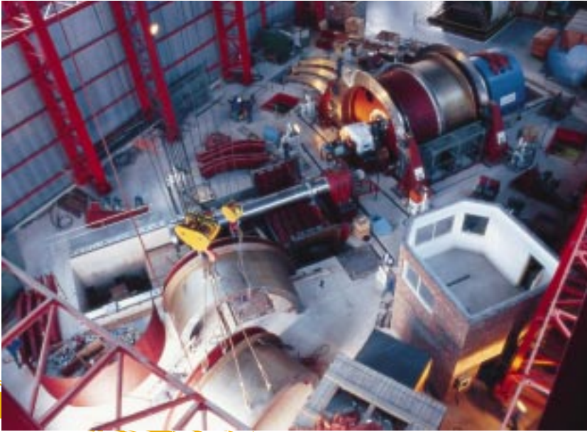
Very sophisticated and highly computerised, the Blair Winder at Moab Khotsong mine will be the deepest single winder in South Africa.
