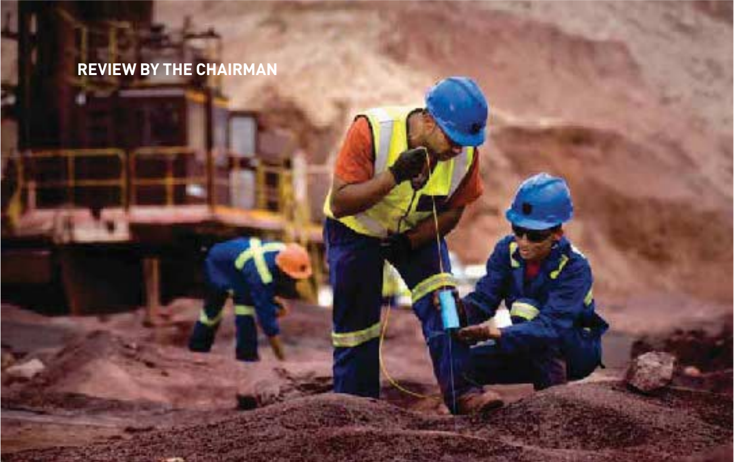
Richard Heyns and Riaan Eilerd, both blasting assistants, preparing to blast at Sishen mine.
