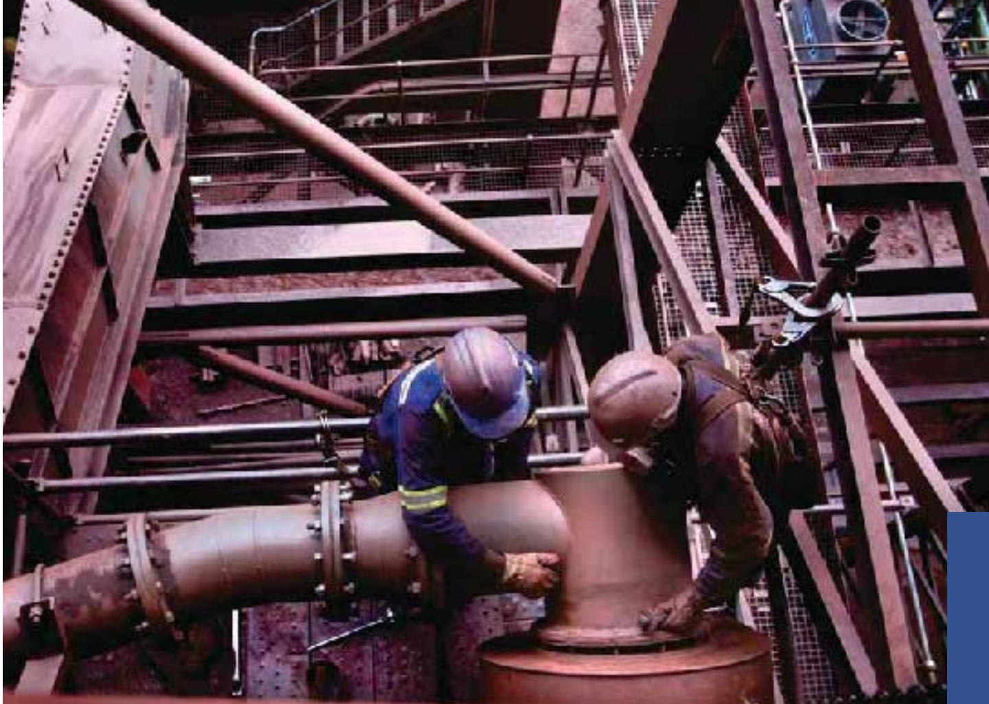
Maintenance workers shifting a pipeline that feeds water to the jig plant at Sishen mine.
