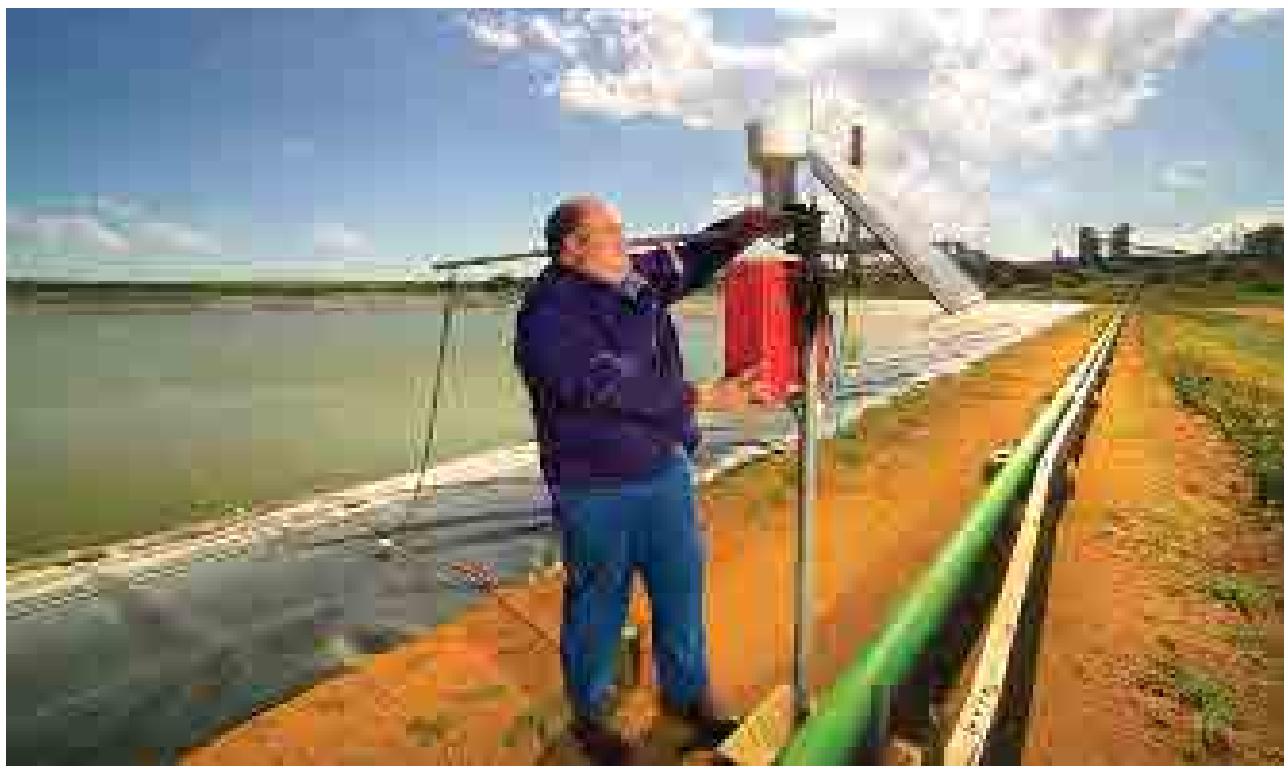
Steve Potgieter, Polokwane Smelter SHE manager, inspecting water monitoring instrumentation at an effluent containment dam.
