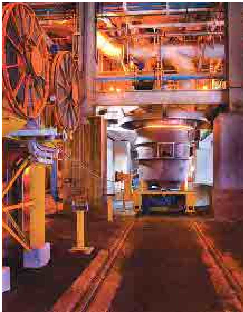
The new fume extraction system on the ladle pre-heaters of the ACP Phase B furnace. Pre-heater fumes are collected and piped, along with other fumes, to the acid plant.
