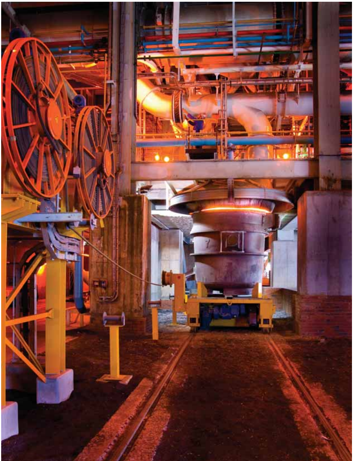
A ladle under the off-gas extraction ducting at Waterval Smelter's ACP plant. The off-gas is sent for treatment at the new acid plant. This system has allowed for improved capturing of fugitive off-gas, thereby reducing the overall SO 2 emissions.
